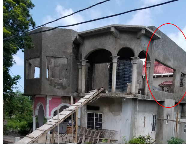
Photo 10: This second story is extremely vulnerable. Not only do the upper walls not align with the bottom walls but construction is extremely irregular and there are very few shear walls. The wall on the right of the building could collapse in high winds if not laterally supported soon.
